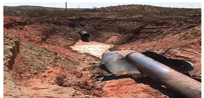
Figure 2. Recent USA Pipeline Failures (8)
