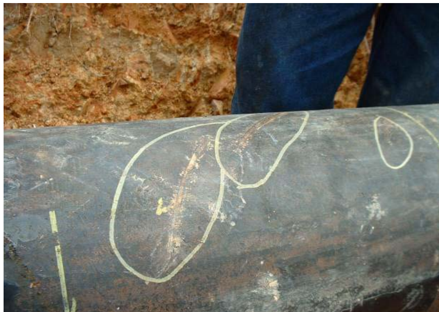
Figure 6 Gouges caused by a back hoe.
