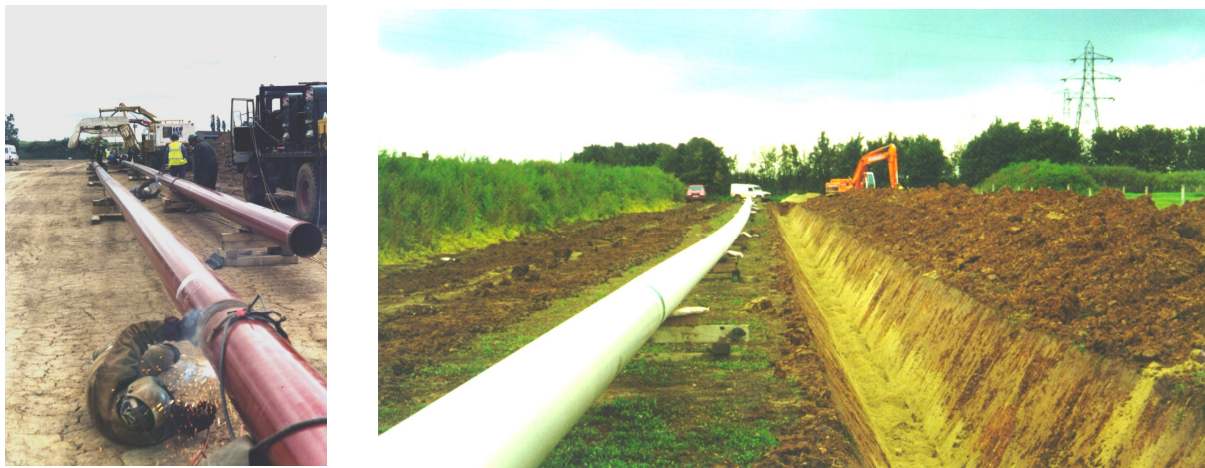
Figure 1. Most of today's oil and gas pipelines are welded together and buried underground
