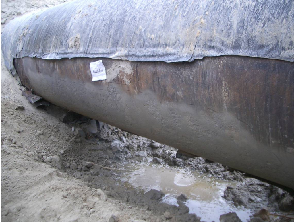
Figure 5 General Corrosion at the Bottom of the Pipe
