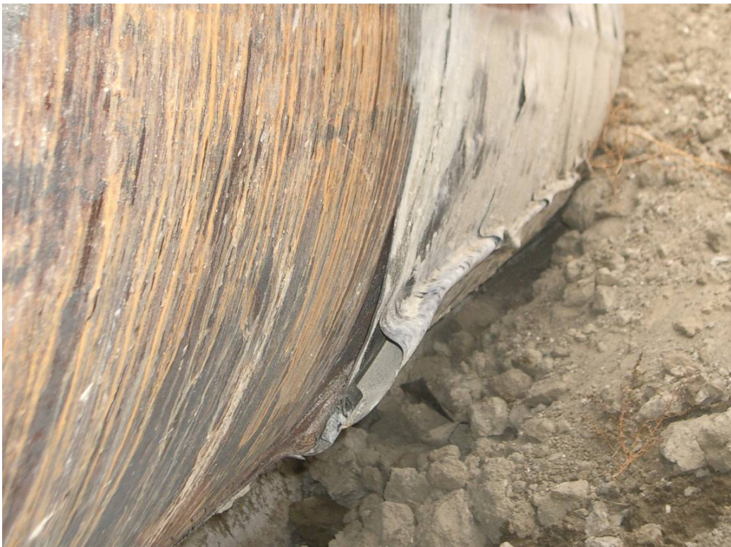
Figure 8 Rucking of a Tape Coating
