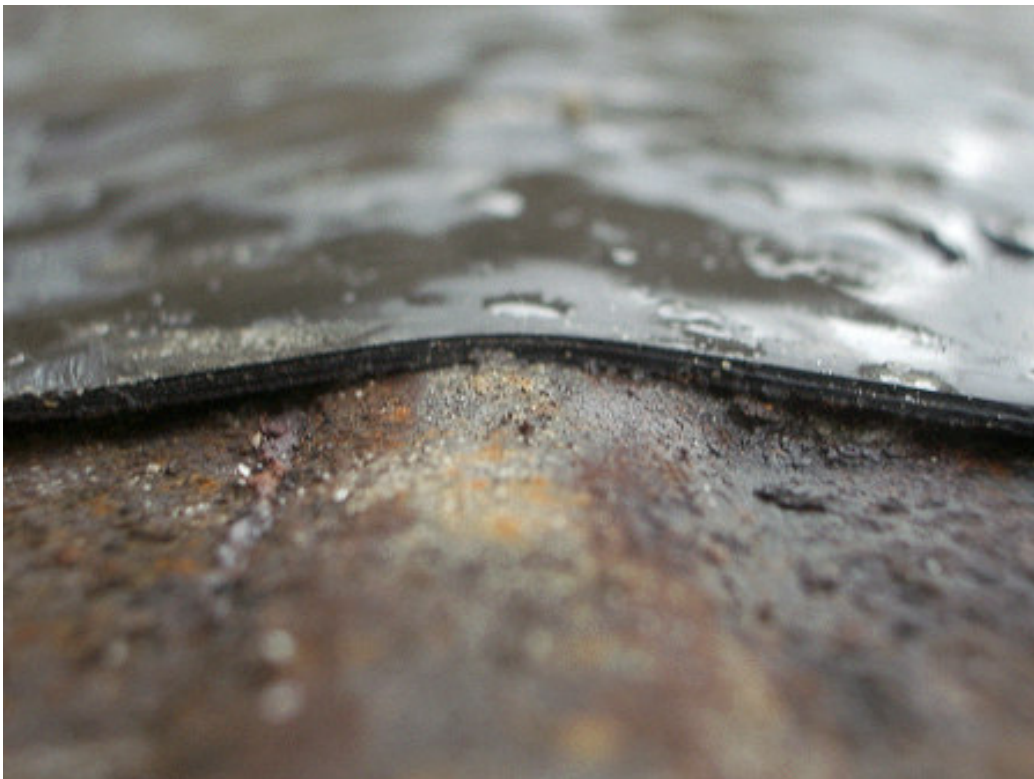
Figure 6 'Tenting' Of A Tape Wrap Coating
