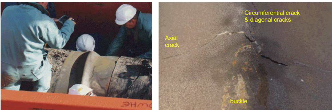
Figure 5. Settlement buckle (taken from The National Transportation Safety Board website: www.nts.gov ).
